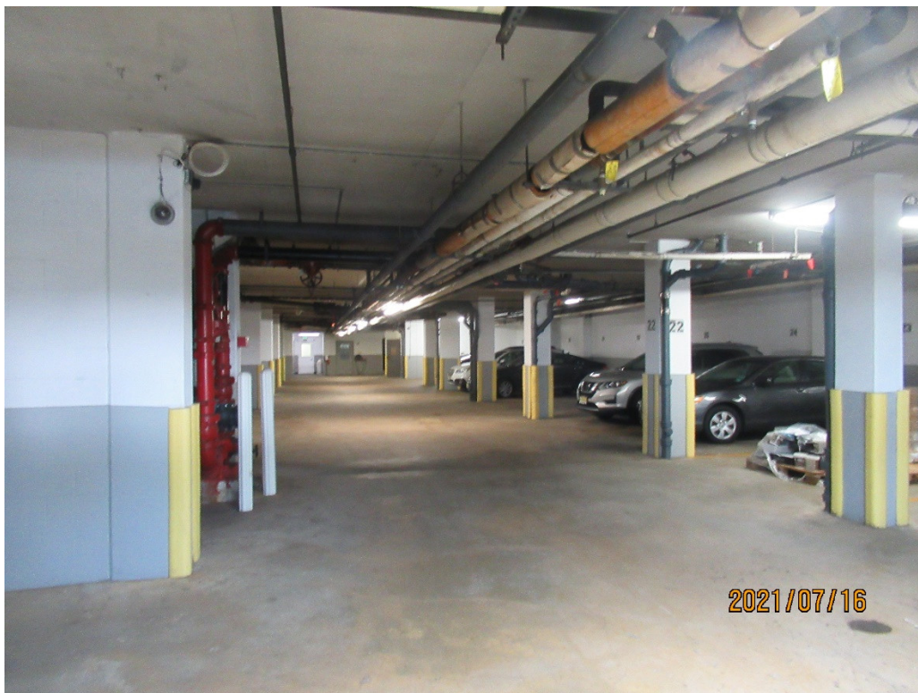
Figure 2. View of Ground Level Parking Garage at Western Half of Residential Tower
