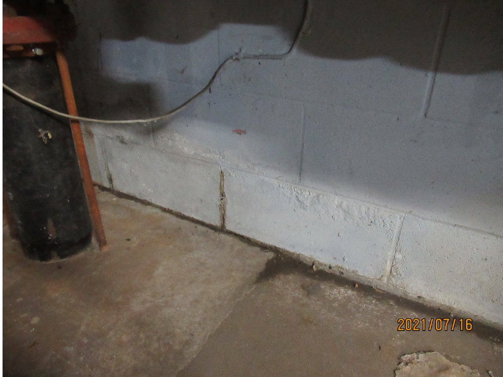
Figure 7. Minor Seepage at Base of West Facing Exterior Wall at Parking Garage
