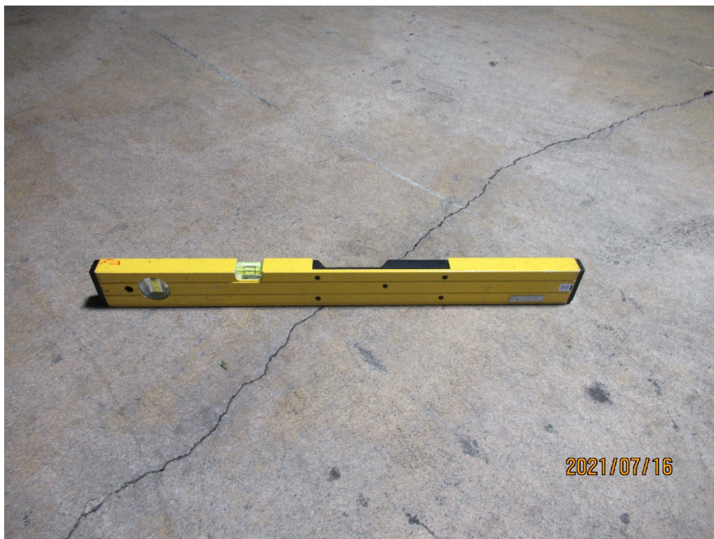
Figure 6. Crack at Ground Supported Concrete Slab at Parking Garage (Note No Vertical Displacement)
