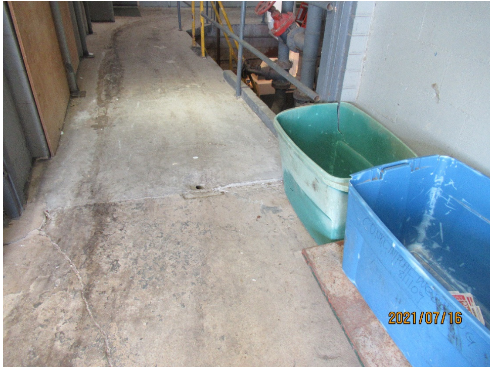
Figure 8. Cracking and Minor Vertical Displacement of Ground Supported Slab at One Story Refuse Room at Northeast Corner of Residential Tower
